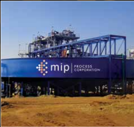
85ft \Phi Thickener in operation
