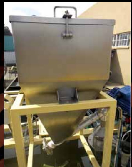
Flocculant hopper and wetting head
