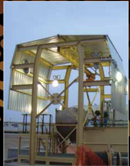
Flocculant Plant with hoist
